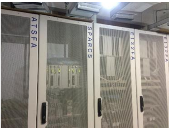
IMAGE : installed SPARCS
