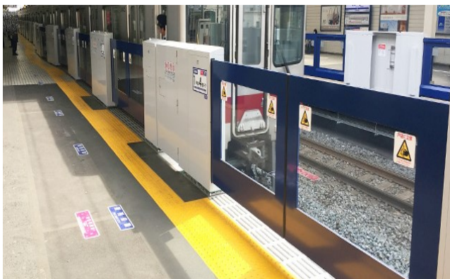
Half Height Platform Screen Doors
